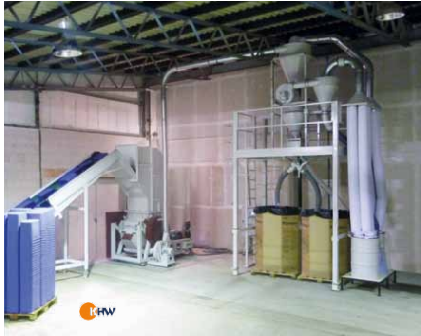
The KHW central system for the creation of regrind with the WITTMANN MC 70-80 granulator, conveyor belt, and filter station.
