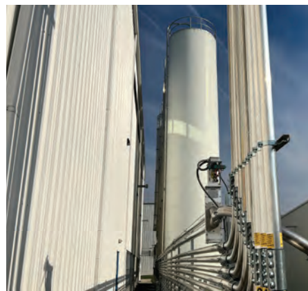
WITTMANN was instrumental in designing and installing new piping and granulators at Monoflo
