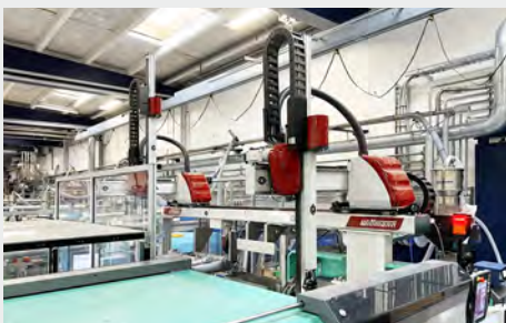
Page 13: SP Moulding (DK) reduces cycle time in production by more than 20%.
